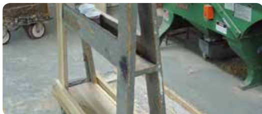
Wood - Splinters and rots
